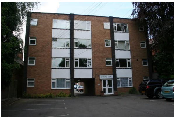
Figure 92. The apartment block in Moseley where we lived for about five months whilst unemployed (photo by AH Field). It appears to now be double glazed.
