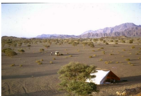
Figure 5 Setting out the power station at Al Mudairib after finally locating the pins
