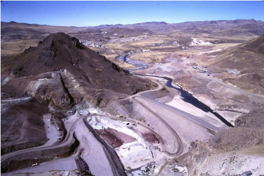
Figure 67 Condoroma dam at an early stage of construction. The red-brown clay forming an impermeable core is being placed over the exposed bedrock.
